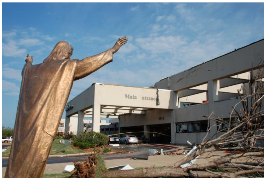
Figure 8: The entrance of St. John's Regional Medical Center after the tornado. (Source: FEMA)
